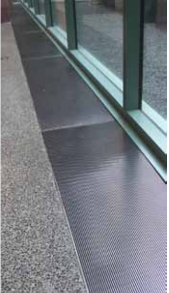
Minneapolis Convention Center Ventilation Grilles
