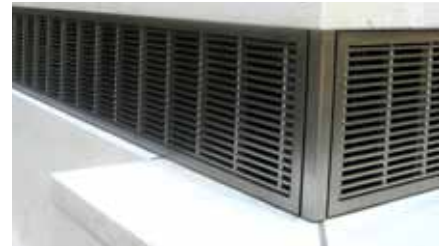
Rittenhouse Condominium Ventilation Grille
